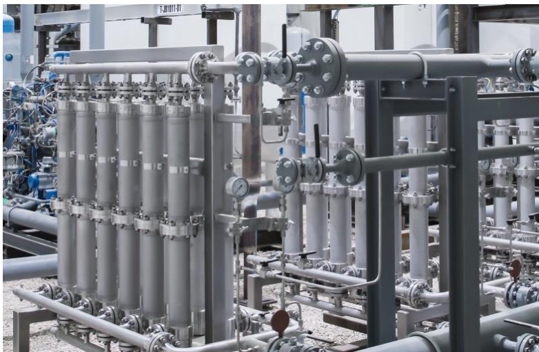
Photo caption: The picture shows membranes – a part of the helium purification facility in Mankota, Canada. (Source: The Linde Group).
